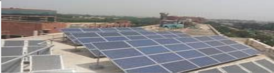
Solar electricity generation Rooftop
