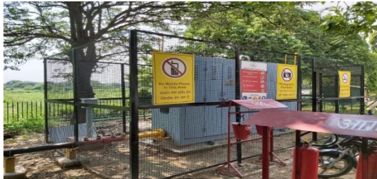
PNG for Boilers/Kitchen.
