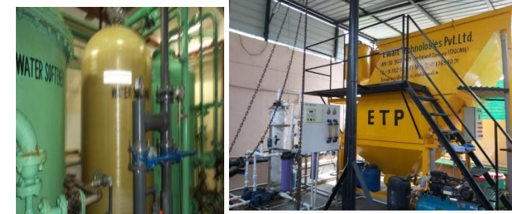
ETP and Re utilization of STP Water
