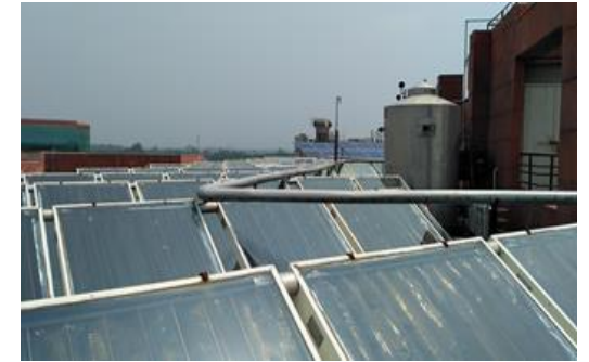
Solar water heating
