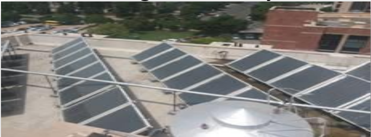
Solar water heating
