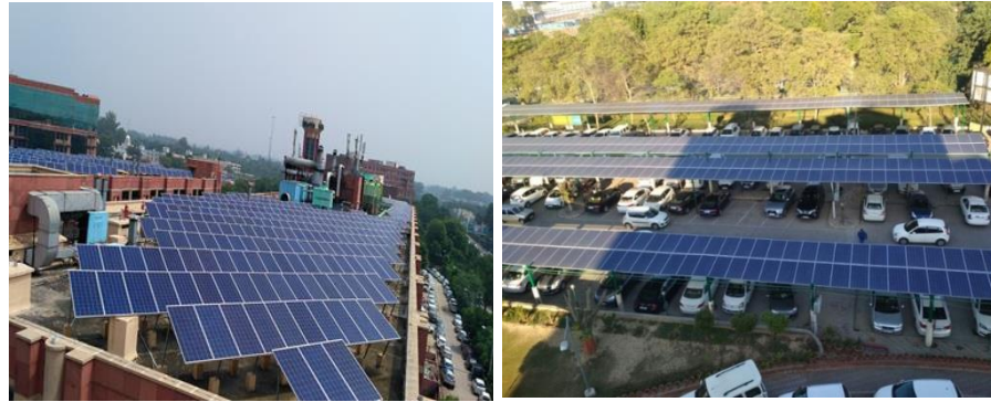
Solar electricity generation
